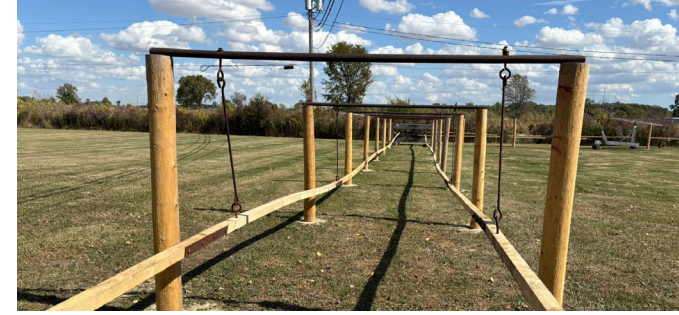
Restoration work completed on the jerker line system at the Oil Museum of Canada.
