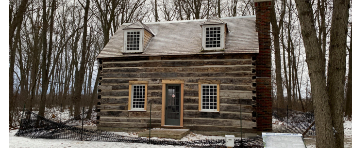
The Canatara Cabin following chinking work, an important step toward sealing and restoring the historic structure.
