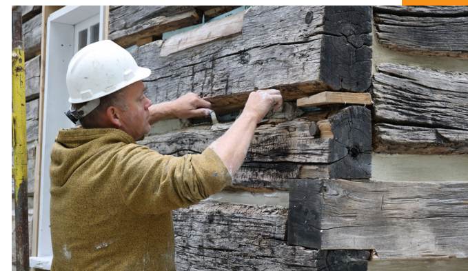
A worker from Bill Dokter Masonry works on chinking the Canatara Cabin as part of restoration efforts.
