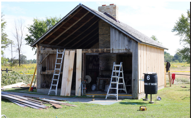
New board and batten being installed on the Blacksmith Shop at the Oil Museum of Canada to help preserve the historic building.
