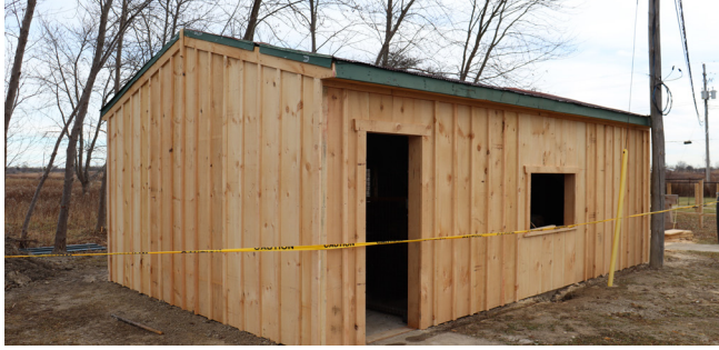
The Chalmers Power House nears complete restoration with new footings and board and batten at the Oil Museum of Canada.
